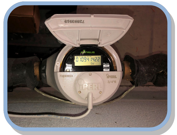
Meter Shown Reading 109,414.22 Gallons
